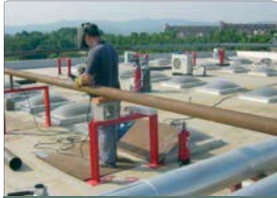
To carry out hot work, an authorisation and complementary safety measures are required.
